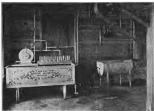
FIG. 1.— Bottle washing machine and sanitary wash tank, showing trap connections. This prevents water from splashing on the floor and soiling clothes or disfiguring machinery. The horizontal pipe should be six inches lower for convenience in stepping over it.
