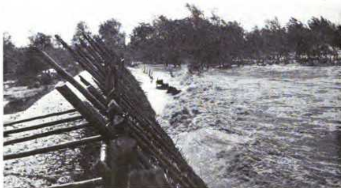
Methods of protection prior to 1916. Earth dam with fascines attacked by waves
